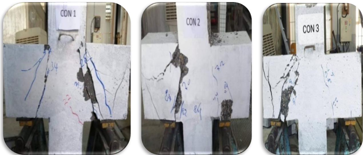
Plate(1) Crack pattern of control corbels (CON1,CON2,CON3)
