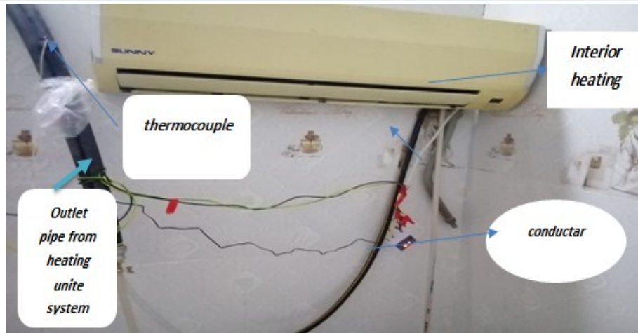
Fig. 3 A Photograph of an Internal Heating System.
